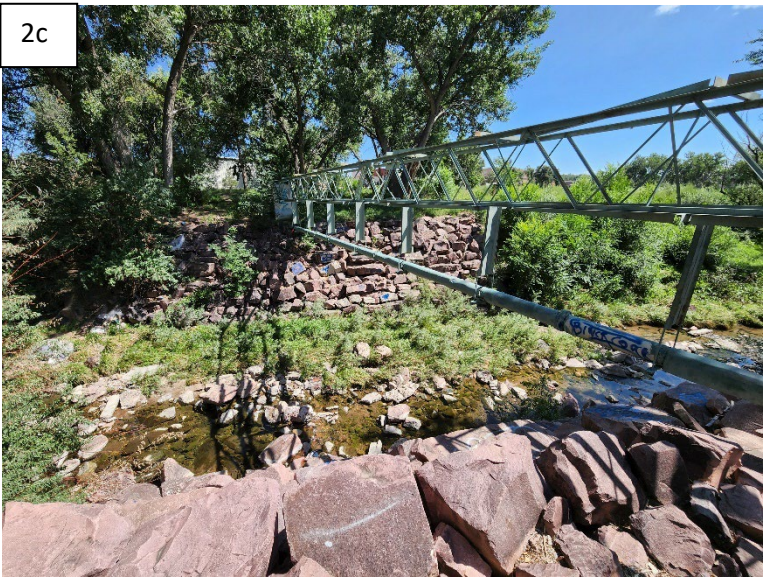
Figure 2a, b and c. The natural banked channel, river incision and erosion of bank, and aerial sewer line
